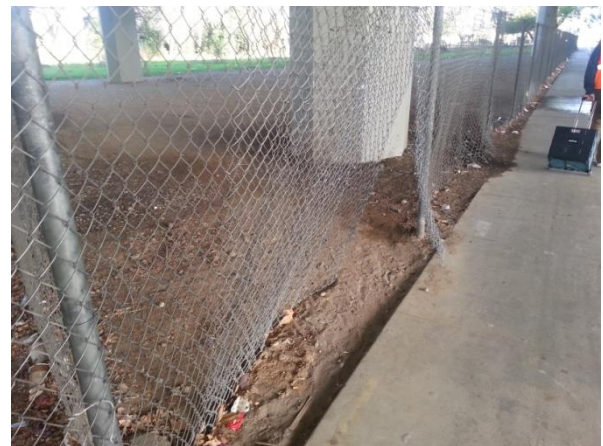
Broken fences encourage trespassing
