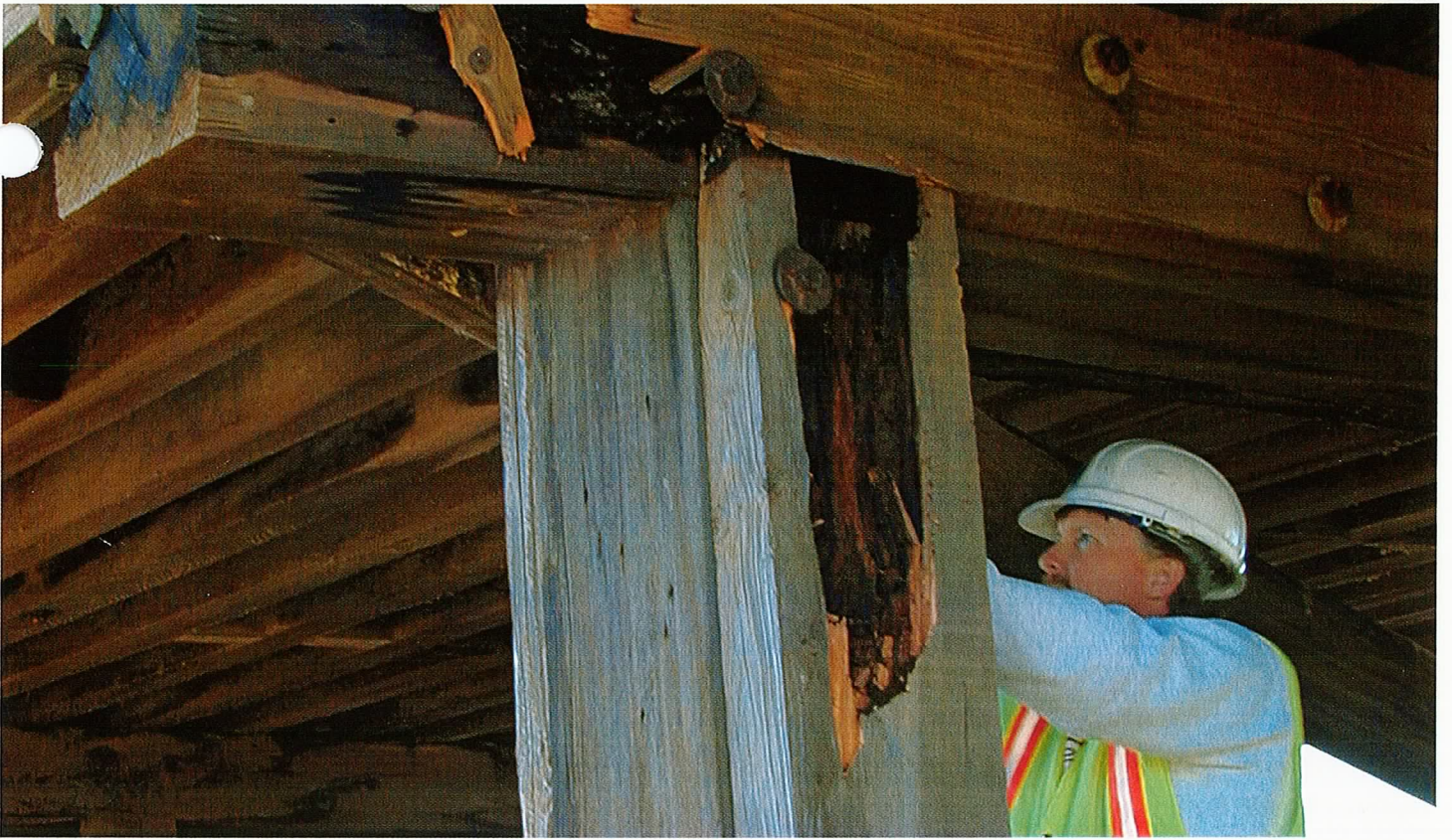
Bent 10 Built-up Section is rotted. 03-SAC-Franklin Blvd, Br#: 24C0155, Mokelumne River Overflow, 02/28/2002, 06B-Dscn0988.jpg
